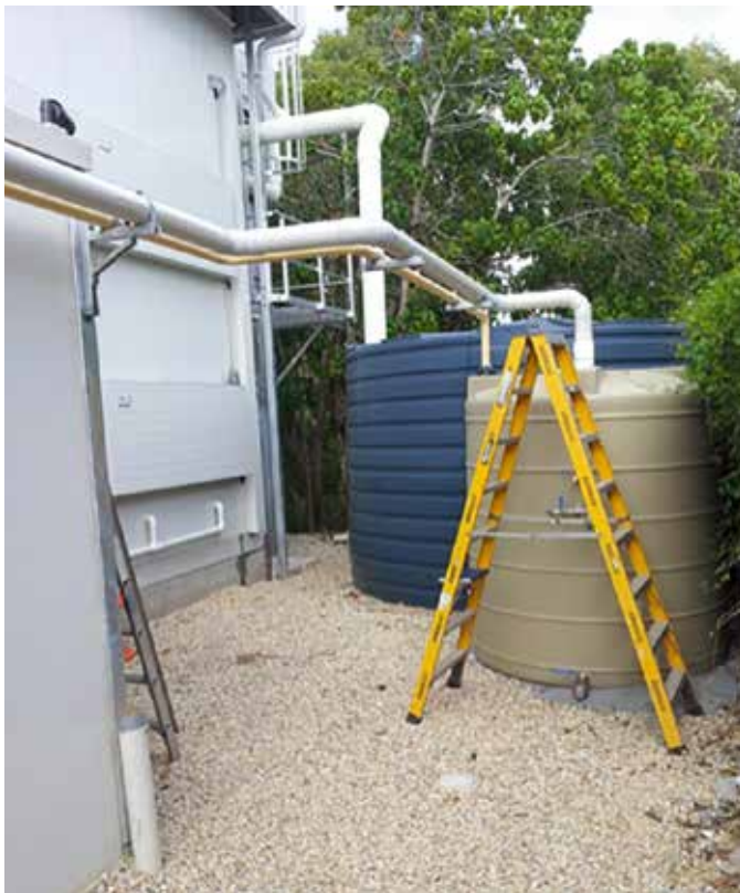
Figure 4: Rainwater storage tank for evaporative condenser make-up water.
